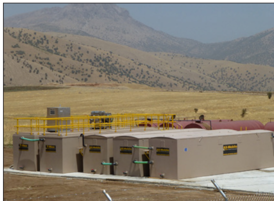
Portable AdvanTex AX-Mobile™ Wastewater Treatment Systems have been installed in remote areas of Kurdistan. They serve 500-person surveying camps.
